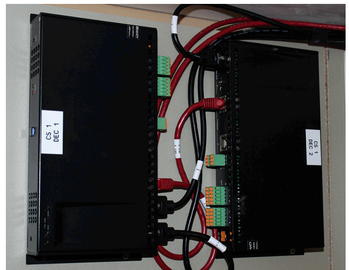
OmniStream decoders mounted discreetly near nursing station displays.
